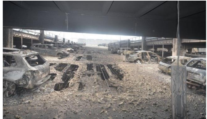
Figure 4: Disintegration of floor slab. Image courtesy of MFRS.
